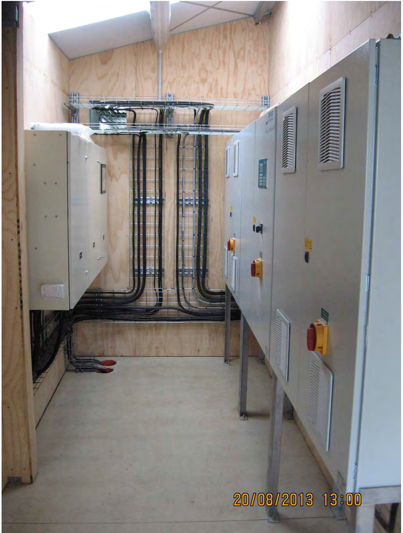
UV Electrical Supply and Control Room
